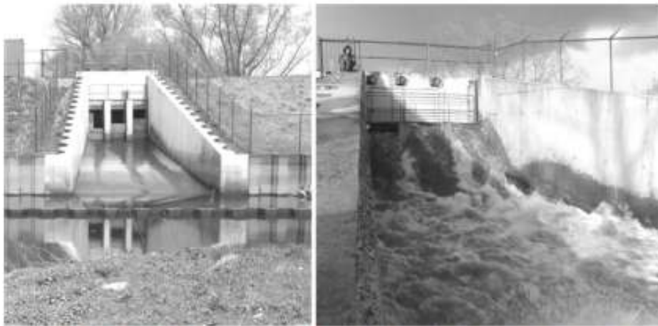
Figure 3. Left: Inlet culvert construction (as seen from within the pilot restoration site), consisting of three inlet culverts, each 1 m wide, with adjustable thresholds at different heights. Right: Close-up of the inlet culverts at spring tide flooding (as seen from within the pilot restoration site).
