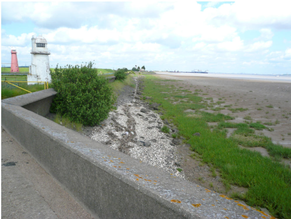
Figure 6.2: Flood Defence Wall along NKM Foreshore
